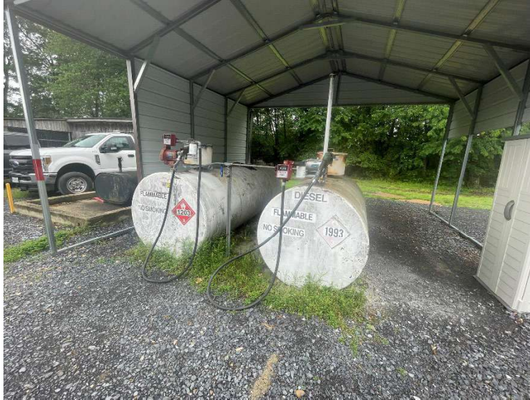
Photograph No. 3 Fuel piping contacting ground in refueling area.
