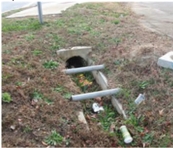
Pipe conveyance filled with vegetation.
