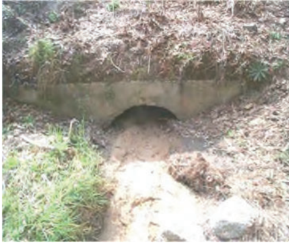
A pipe filled with sediment, inhibiting flow.
