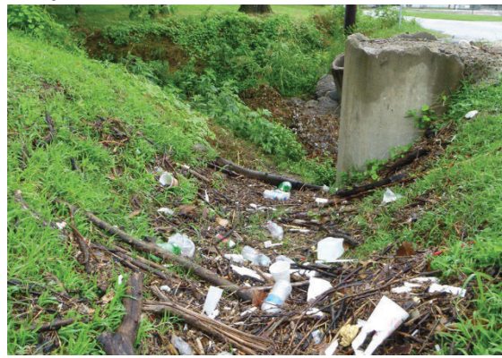
Litter and debris within a swale.
