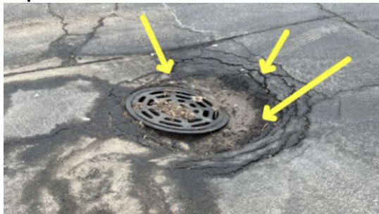
Failing asphalt surrounding the inlet
