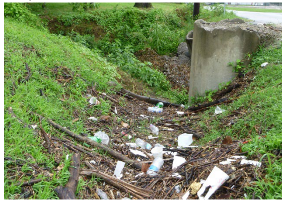
Litter and debris within a swale.
