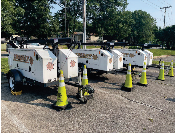
Photograph No. 1 Portable generators (3) stored on site outside.
