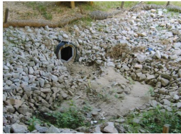
Sediment accumulation at swale inlet.
