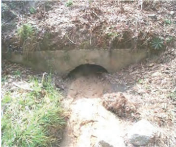
A pipe filled with sediment, inhibiting flow.
