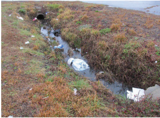
Litter and debris within a ditch.
