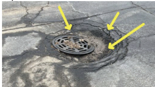
Failing asphalt surrounding the inlet
