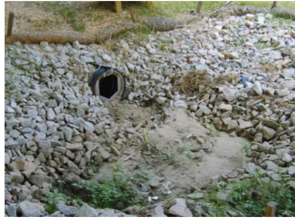
Sediment accumulation at swale inlet.
