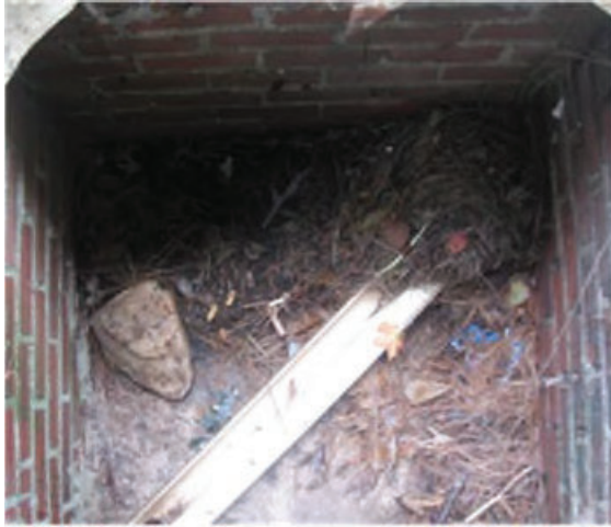
Sediment and debris inside stormwater inlet
