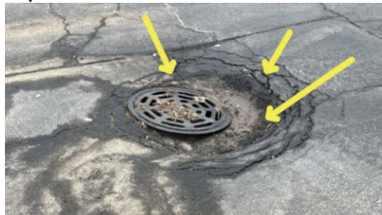
Failing asphalt surrounding the inlet
