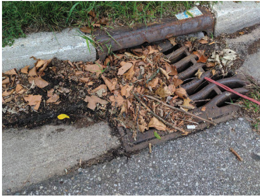
Debris and sediment blocking inlet/catch basin grate.
