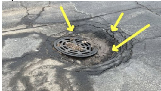
Failing asphalt surrounding the inlet
