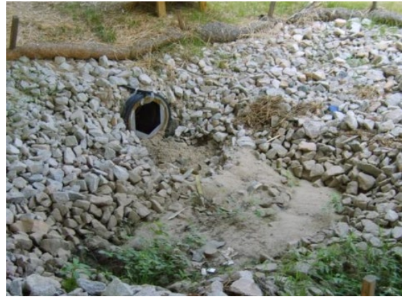
Sediment accumulation at swale inlet.
