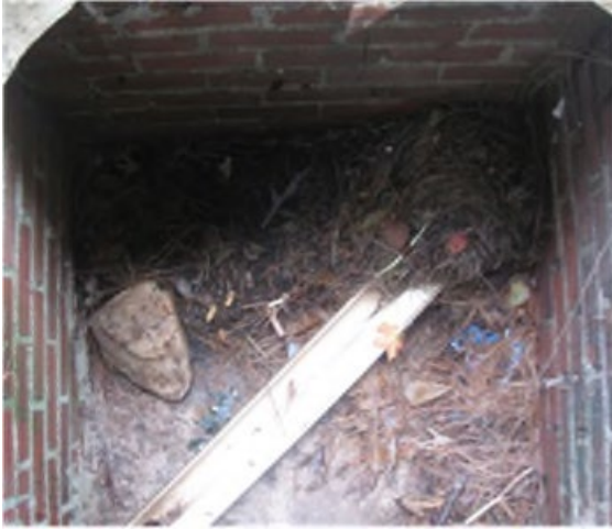
Sediment and debris inside stormwater inlet
