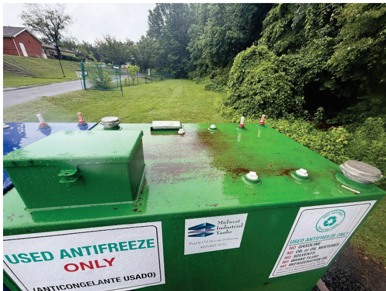
Photograph No. 4 Tank top view of the 500-gallon double-walled used antifreeze AST.
