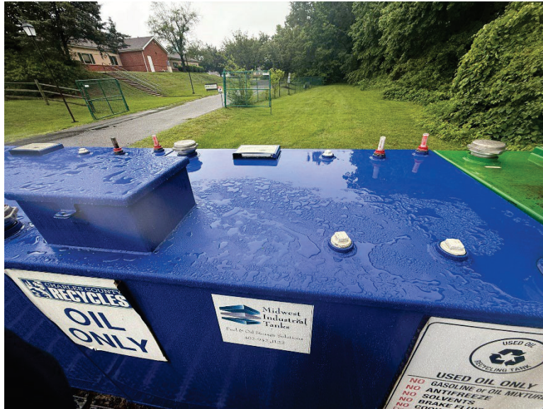
Photograph No. 3 Tank top view of the 500-gallon double-walled used oil AST.
