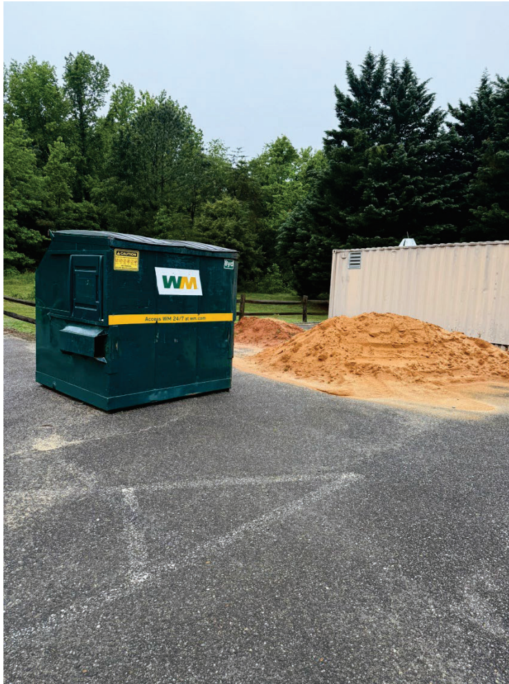
Photograph No. 1 Sand pile stored with no buffer protection.
