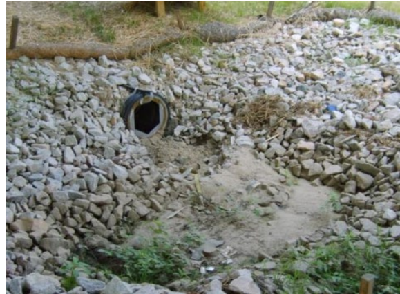
Sediment accumulation at swale inlet.
