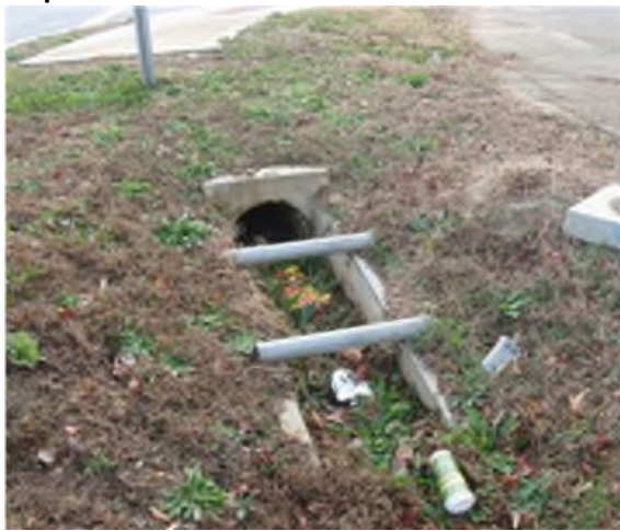
Pipe conveyance filled with vegetation.
