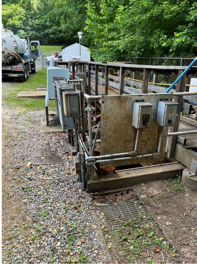
Photograph No. 2 Clogged trench grate adjacent to Blower 1.
