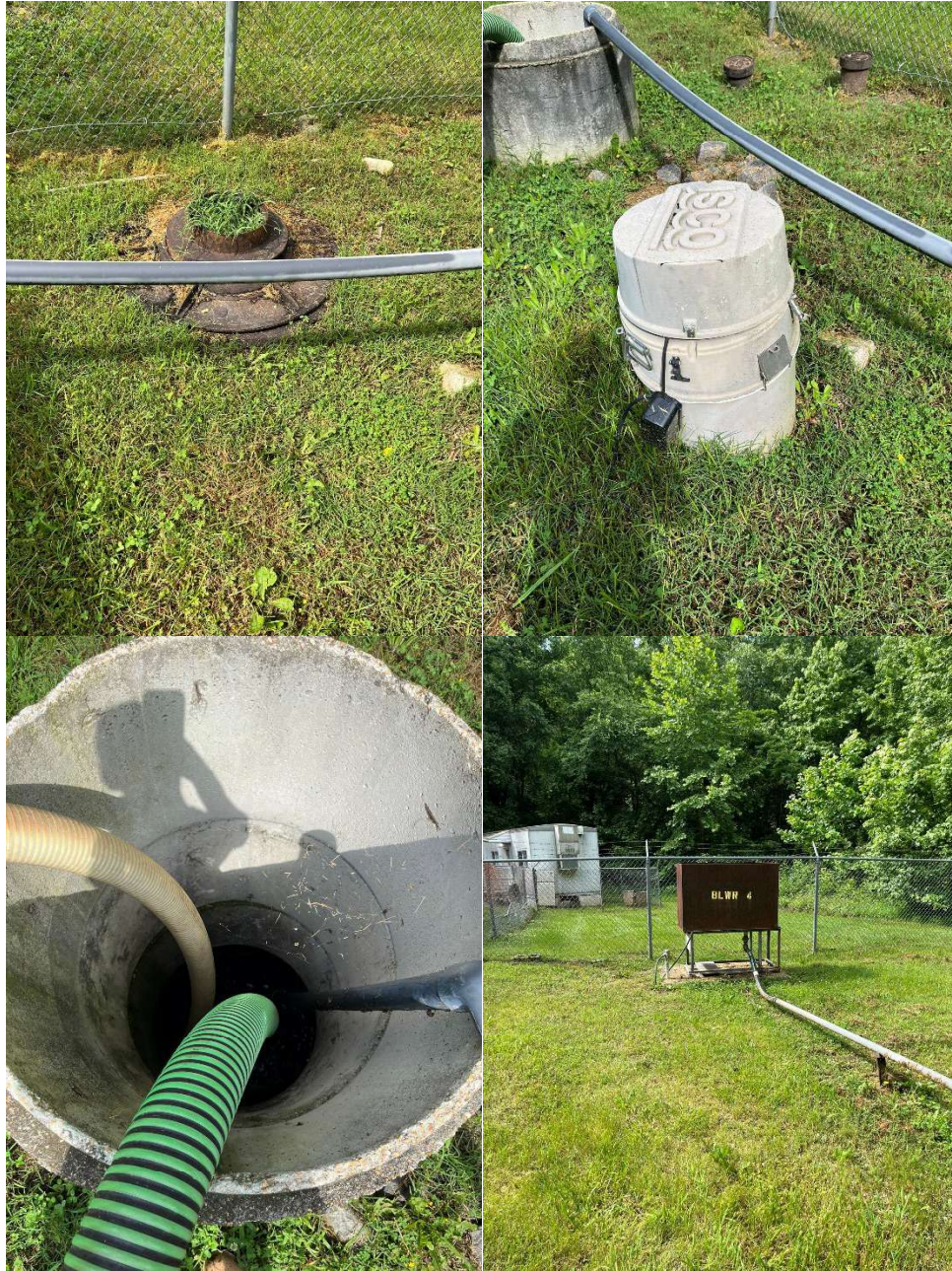
Photograph No. 3, 4, 5, & 6 Piping around the facility.
