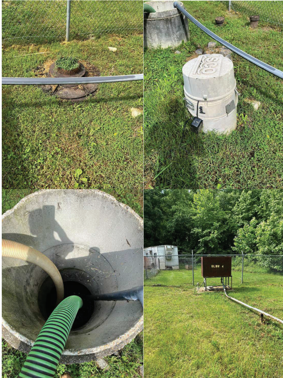
Photograph No. 3, 4, 5, & 6 Piping around the facility.
