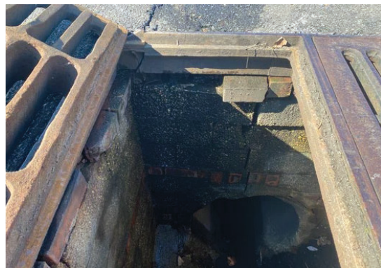
Failing brick walls with a stormwater inlet.
