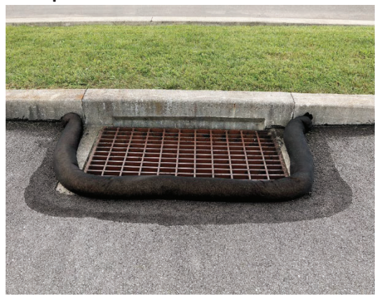
Example of an inlet filter sock, replace if damaged.
