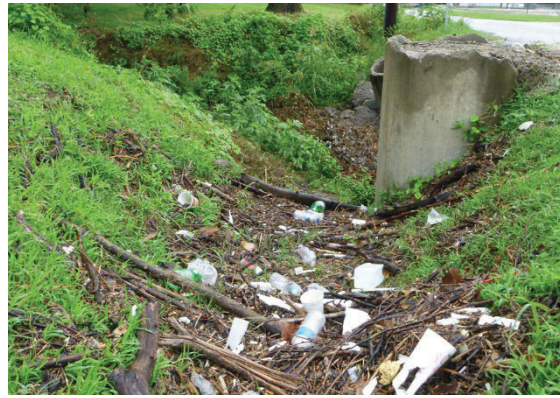
Litter and debris within a swale.
