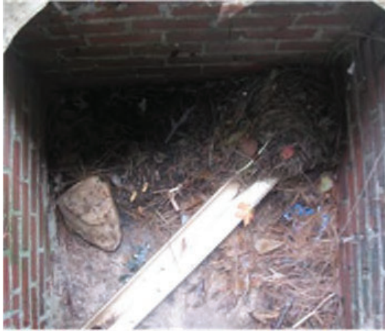
Sediment and debris inside stormwater inlet
