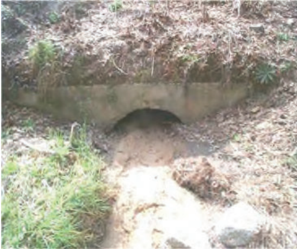
A pipe filled with sediment, inhibiting flow.
