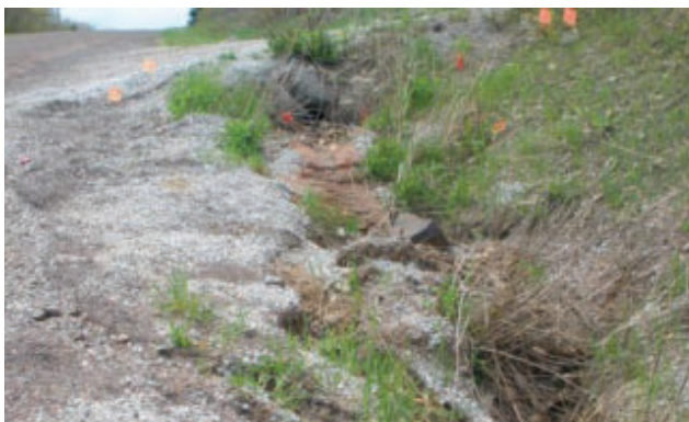
Erosion and slumping within a drainage ditch.
