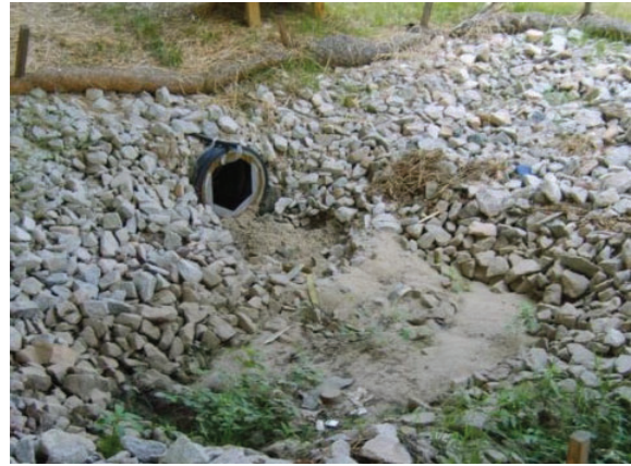
Sediment accumulation at swale inlet.
