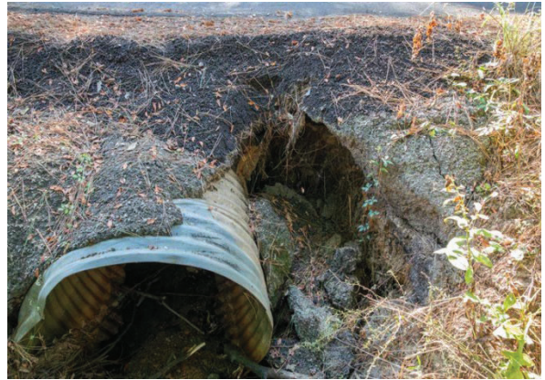
Evidence of erosion around a culvert.
