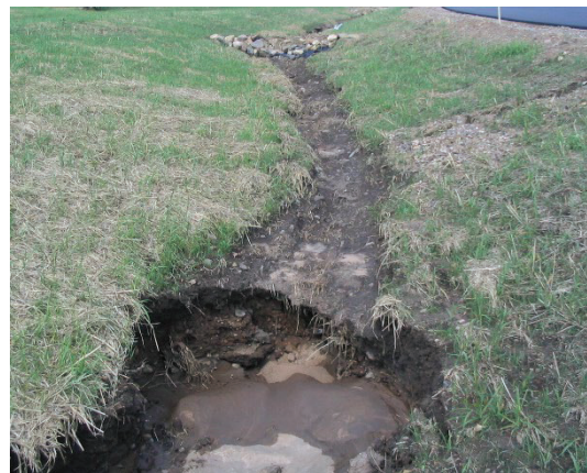
Slumping within a drainage swale.
