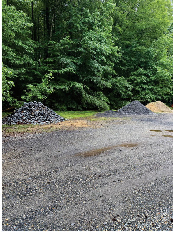
Photograph No. 5 Sediment stockpiles stored on site.
