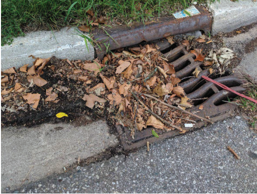
Debris and sediment blocking inlet/catch basin grate.
