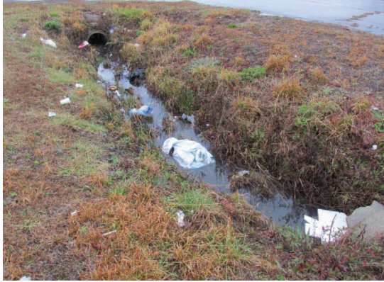
Litter and debris within a ditch.
