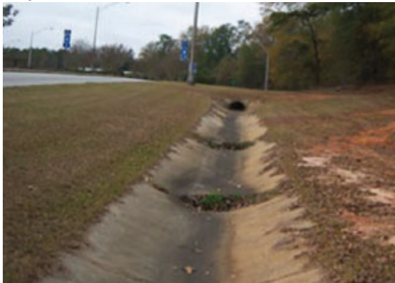
Cracks and joint separation in concrete channels, removal of vegetation may prevent future damage.
