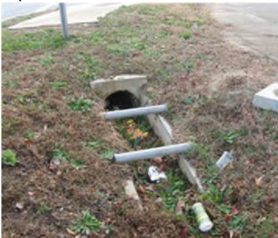
Pipe conveyance filled with vegetation.
