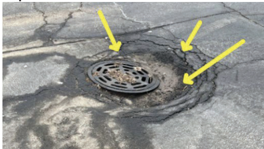
Failing asphalt surrounding the inlet
