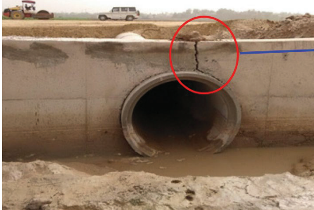
A crack in the culvert headwall.
