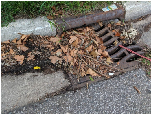
Debris and sediment blocking inlet/catch basin grate.
