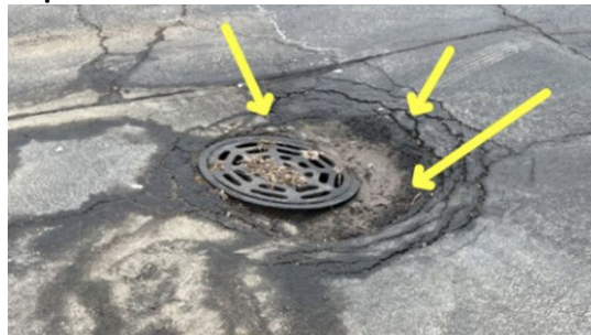
Failing asphalt surrounding the inlet
