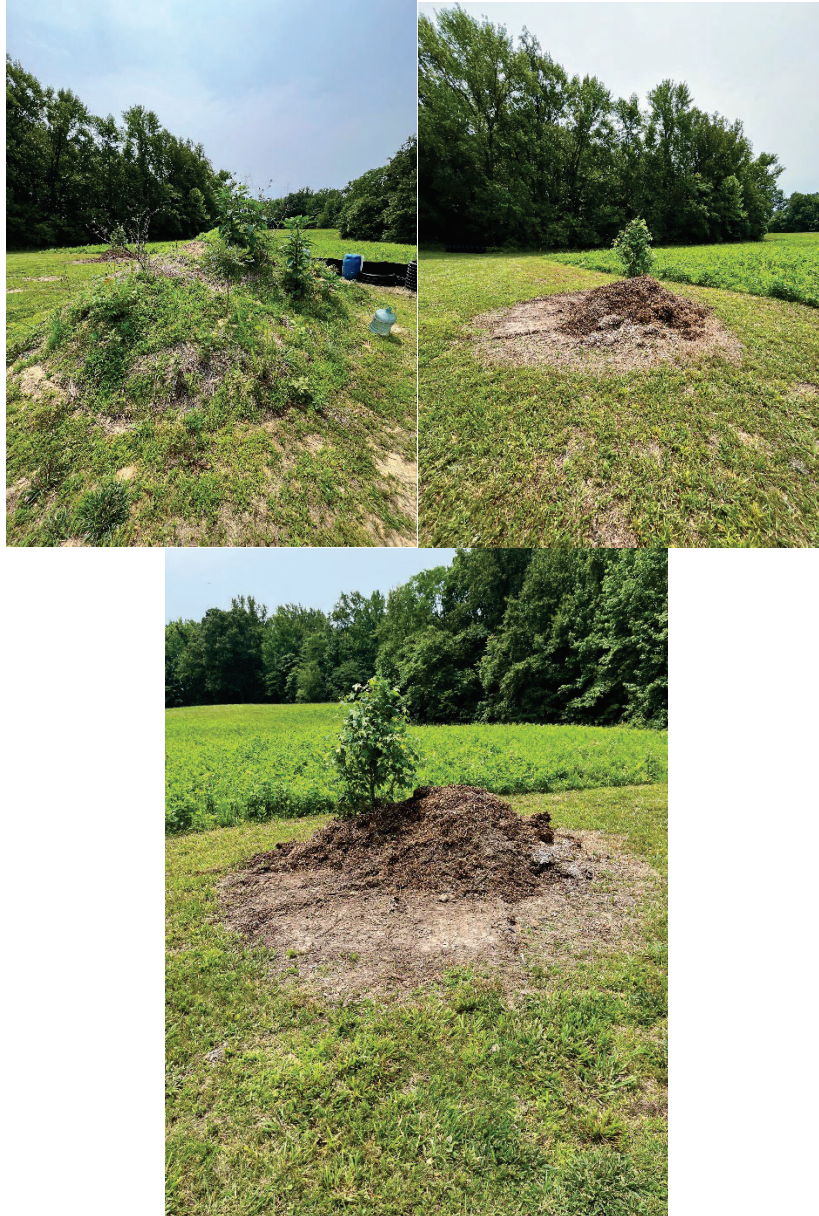
Photograph No. 4, 5, & 6 Sediment storage on-site without sediment fencing.
