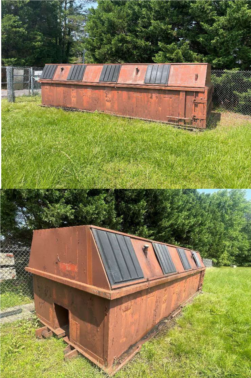
Photograph Nos. 4 & 5 Secondary containment system for ASTs with missing labels and visible corrosion.
