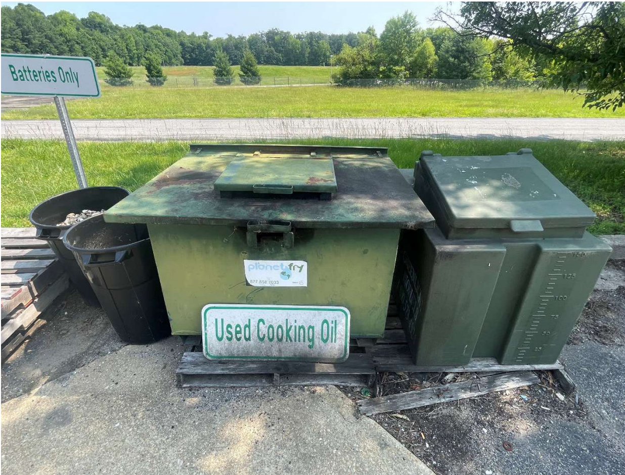
Photograph No. 6 ASTs used for citizen drop-off of used cooking oil with faded and missing labels.
