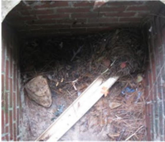
Sediment and debris inside stormwater inlet
