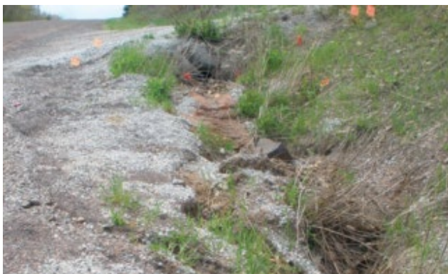
Erosion and slumping within a drainage ditch.
