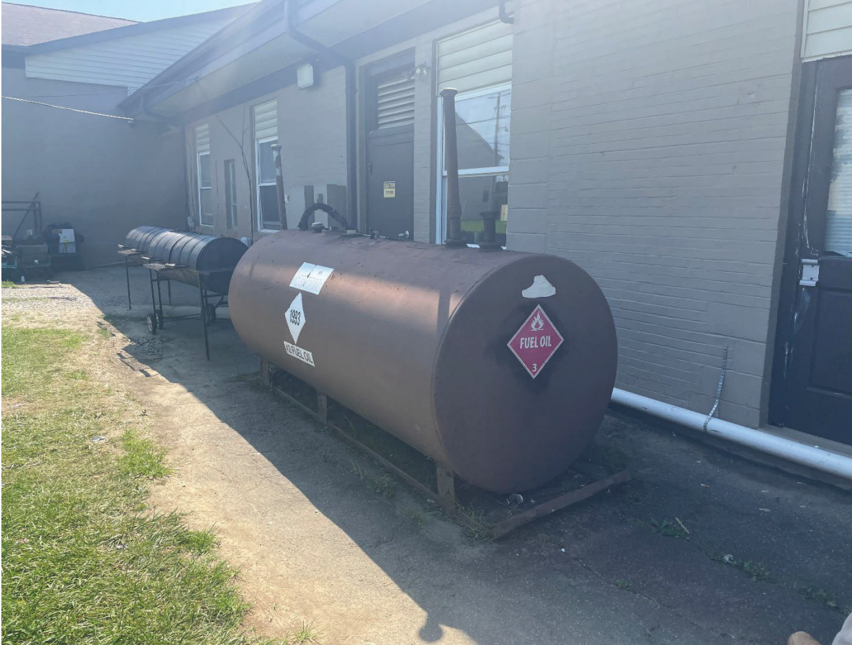
Photograph No. 3 Aboveground fuel oil storage tank with faded labels.
