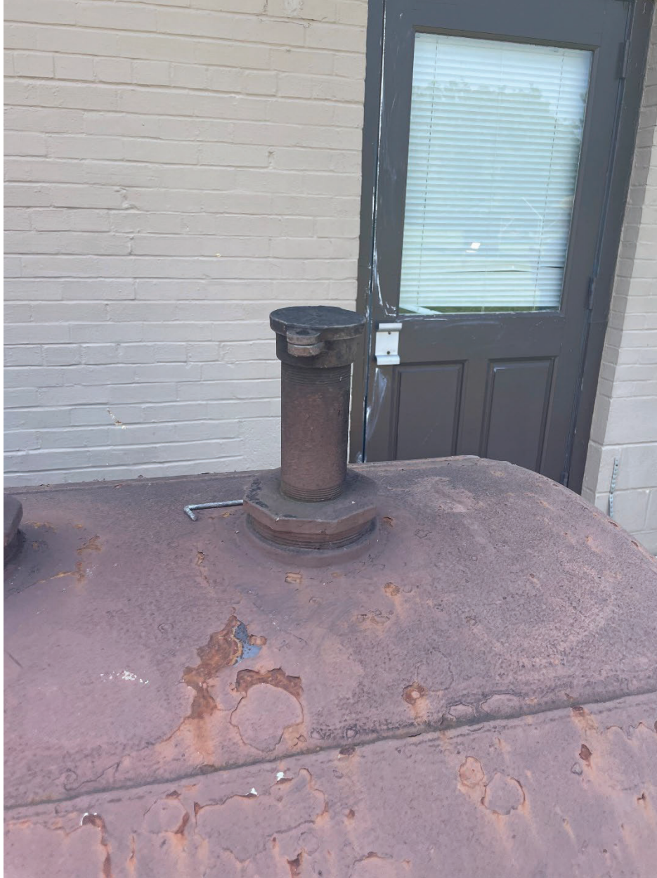
Photograph No. 4 Vent of aboveground fuel tank, with lock on fill port missing.
